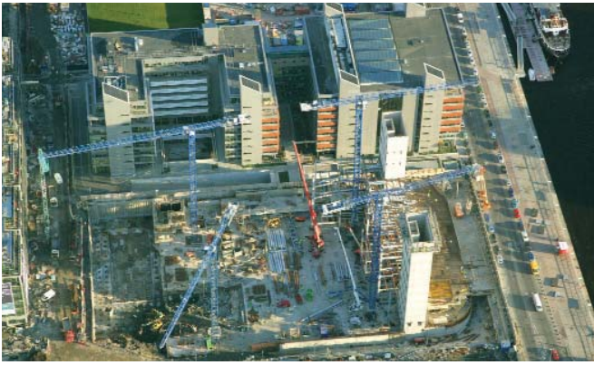
3 Aerial view showing basement works and steelwork erection in December 2007 ©Peter Barrow Photographers
