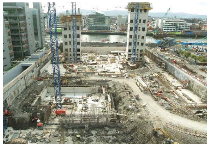
2 View from office block to the North of the site, showing basement works in September 2007 ©Peter Barrow Photographers
