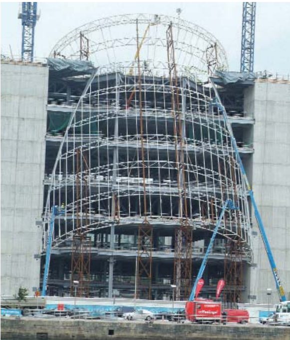
9 Front elevation of building, during July 2008, showing completed 'drum' structure ©Peter Barrow
