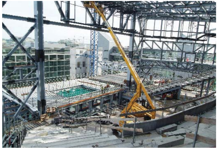
4 The inside auditorium looking North, showing steelwork erection during August 2008 ©Peter Barrow Photographers
