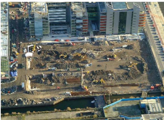
1 Aerial view, taken in January 2007, of site plate with secant piling works ©Peter Barrow Photographers
